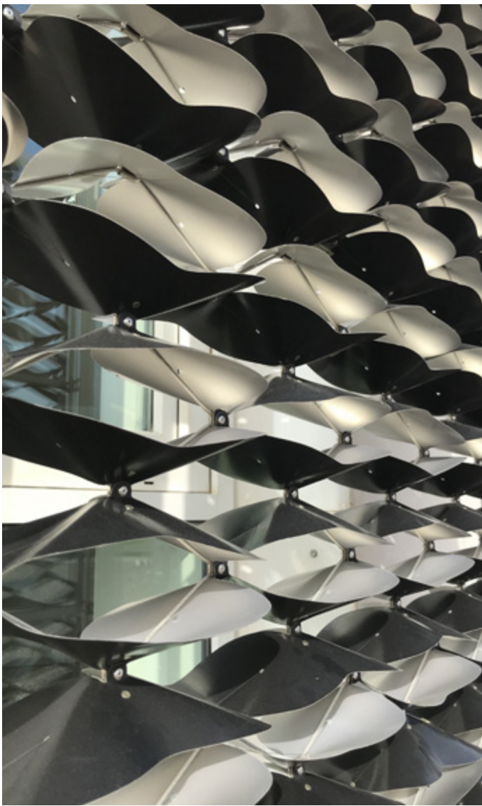
Installation of Adaptex Wave Shading System at GUTech Eco House in Muscat. Photo: Maxie Schneider
